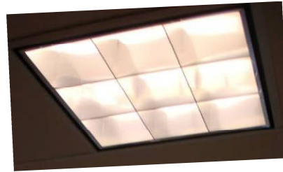
Existing Fixture 27 Foot Candles ~90 Watts
