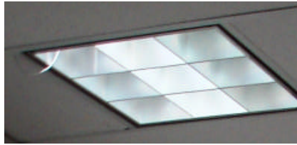
LED Retrofit 57 Foot Candles ~35 Watts
