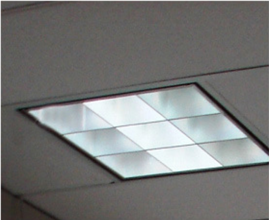
AFTER LED INSTALLED LED Retrofit Neutral White ~40 Foot Candles ~20 Watts
