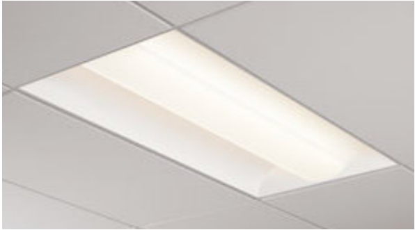
AFTER LED INSTALLED Acrylic Diffuser
